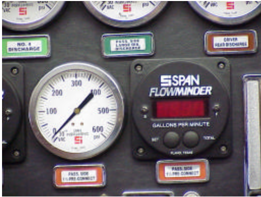
Figure 13: Outlet pressure gage with Flow gage for discharge outlet.
